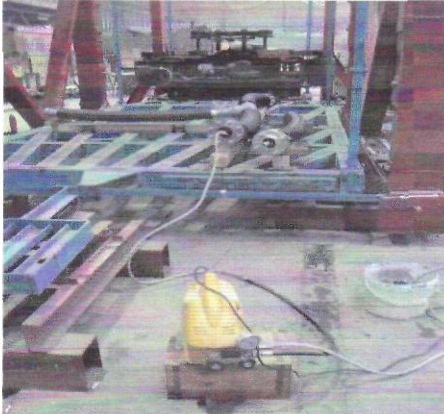
Fig. 3.2. The general view of the pipelines installed on the vibroplatform
