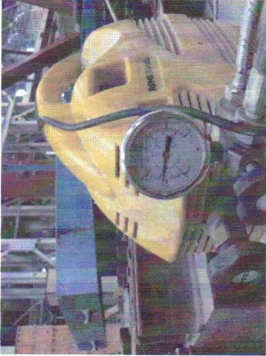
Fig. 6.4. Pumping station for pipeline pressure determination (on the scale of 1.1 bar)
